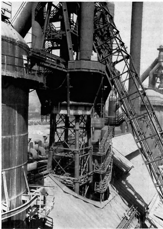
Fig. 7: Erection scaffold for supporting the blast furnace top after dismantling the old stack mantle
