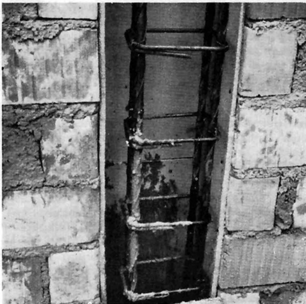
Fig. 7: Recesses for supports lined with 1 cm thick insulation slabs and support armoring placed in position
