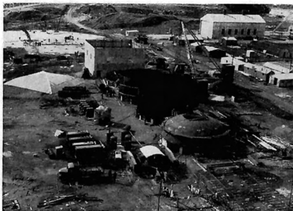
Fig. 10: Welding of the pressure vessel for the reactor at Calder Hall — in the background protective construction with its roof removed
