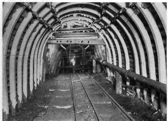
Fig. 4: Pit head winch compressed air feeding line in a shaft provided with steel rings
