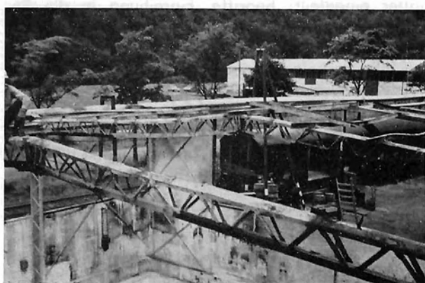
Fig. 1: Reconstruction of an Accumulator-Storage Shed, 3 hours after fire (works photo)
