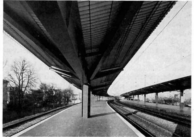
Fig. 39: Prestressed steel wire roof for a local railway station in Vienna (Schnellbahnstation Floridsdorf); anchoring
