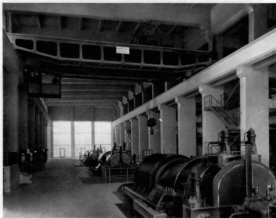
30-t-crane Power Station St. Andrä, of modern, welded steel construction
